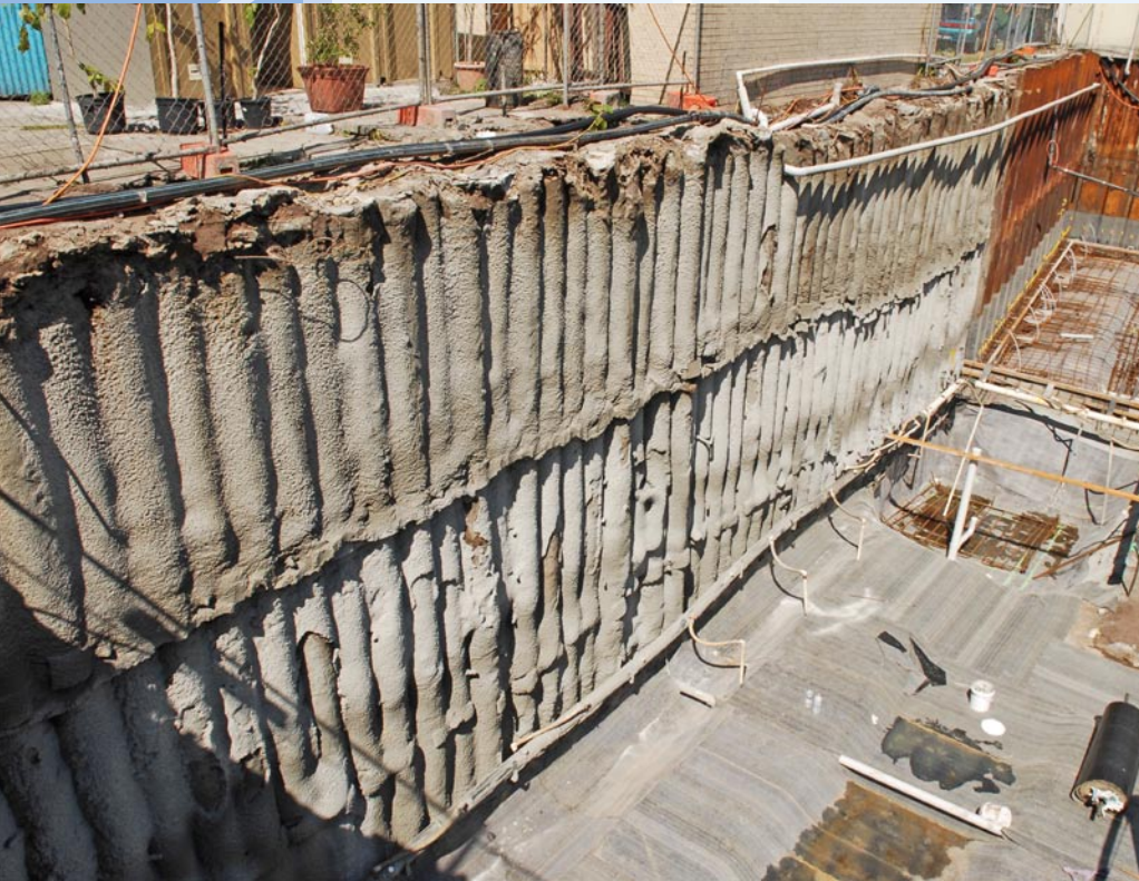
Above: CFA piles demonstrate their value in extremely close proximity to an occupied neighbouring dwelling.
