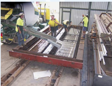
Far right and inset: Replacement of a decades old section of revetment wall at Pacific Fair, Gold Coast.
