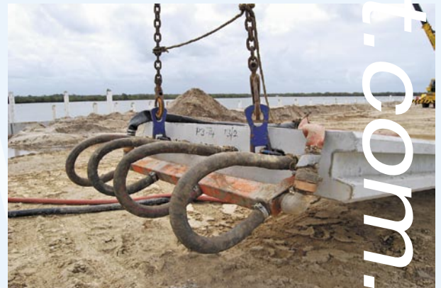
Above: The water jetting head attached to the top of the panel prior to lifting.
