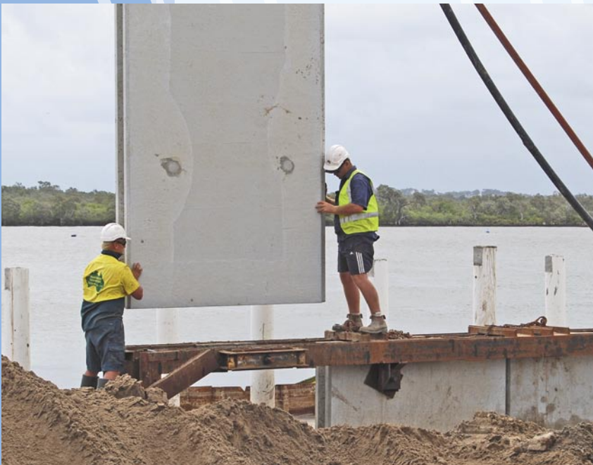
Left: Lifting a panel to the revetment line. The capping beams that top the wall can be seen in the foreground.
