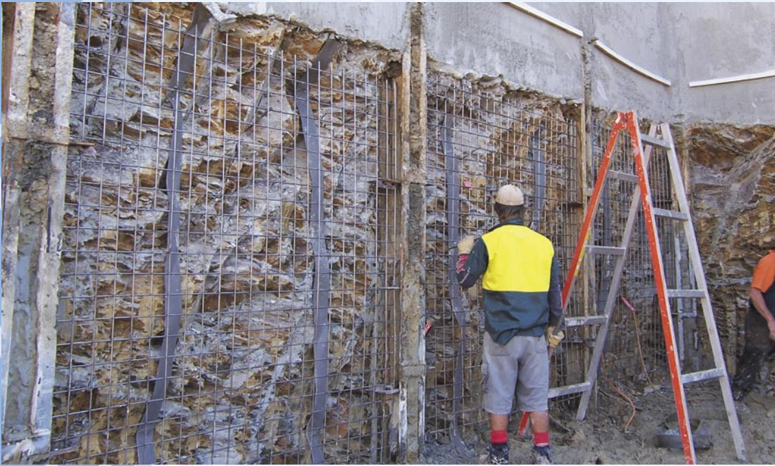
Above: The use of a soldier pile wall to a clay and rock profile excavation.
