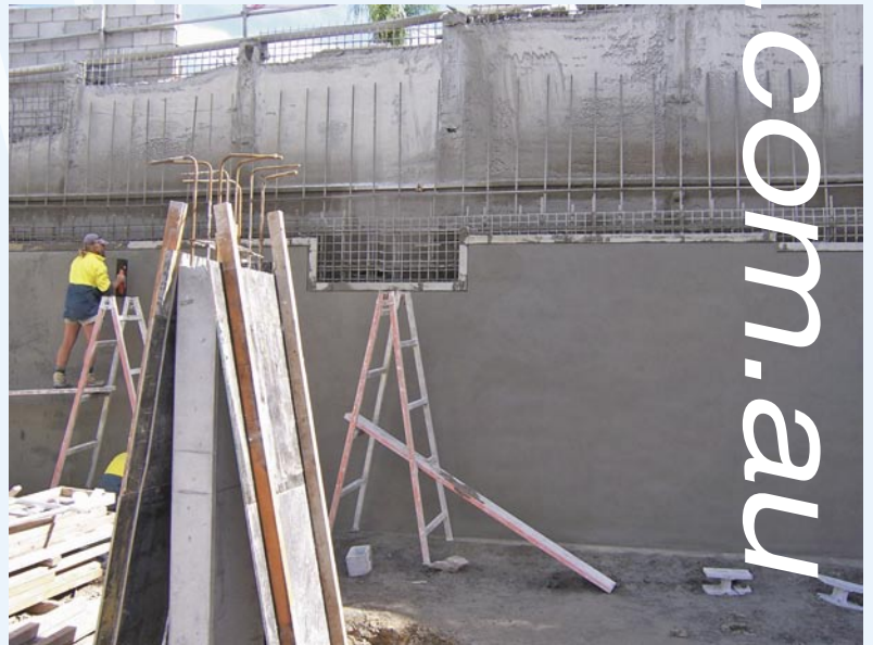
Right: Shotcrete being applied as a finished wall over a soldier pile wall.
